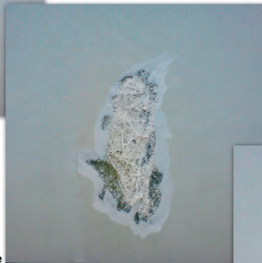
Diagnostic finding at repair: dry laminate
